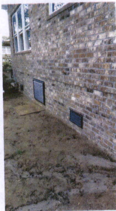
LARGE VENT AND SMALL VENTS
