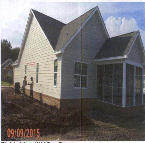
Right side HVAC Rear
