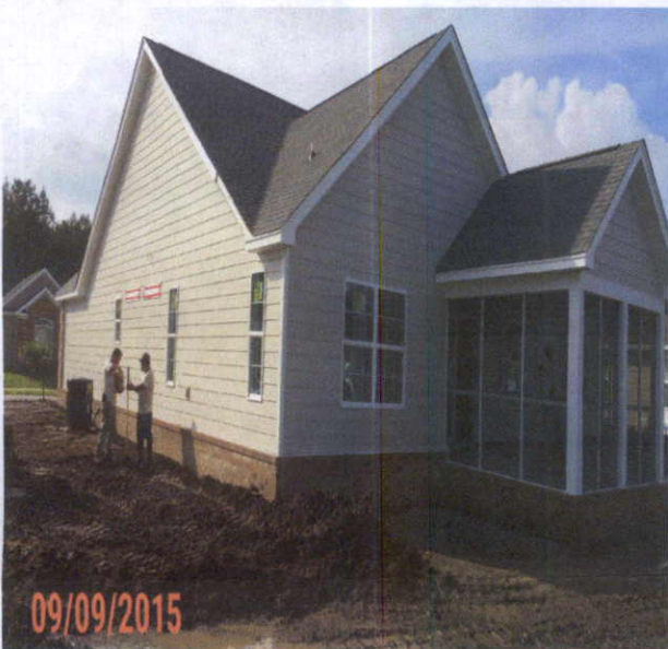
Right side HVAC Rear
